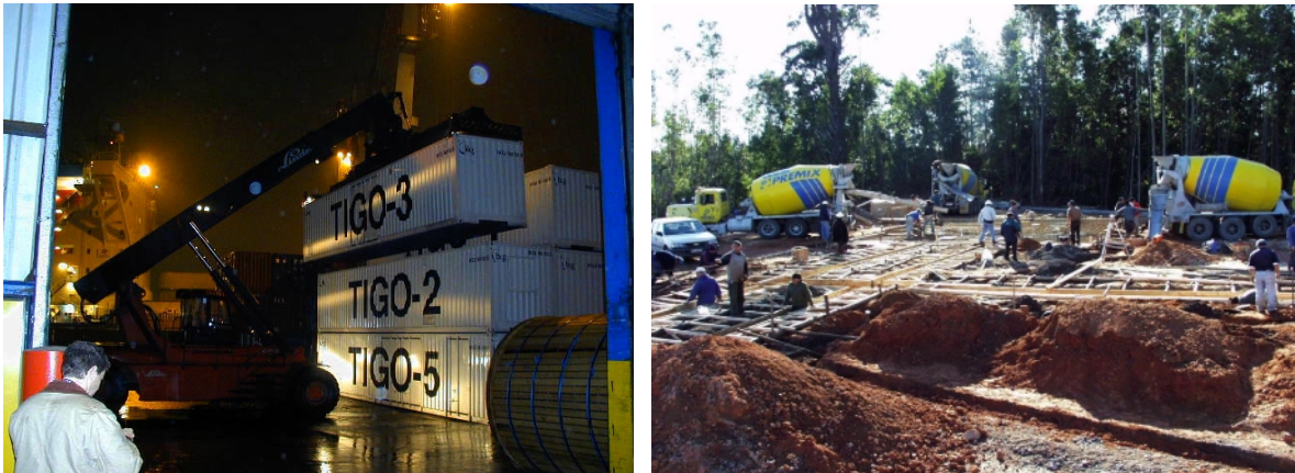
Figure 4.1-14 (left): The TIGO six pack (six containers) during loading onto the ocean vessel; (right): The platform for hosting the TIGO containers in Concepcion under construction.
