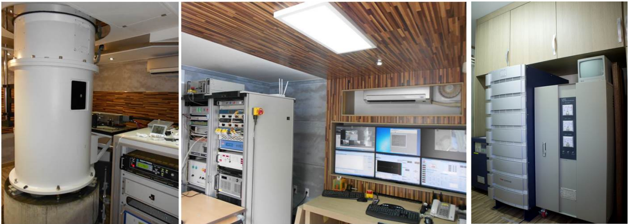
Figure 3. Internal Structure of ARGO-M, laser room(left), operation room(middle), accessory room(right)
